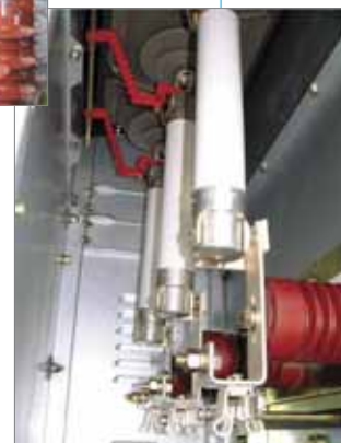
internal view of service compartment for transformer protection units
