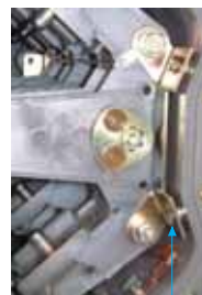
internal earthing connection
